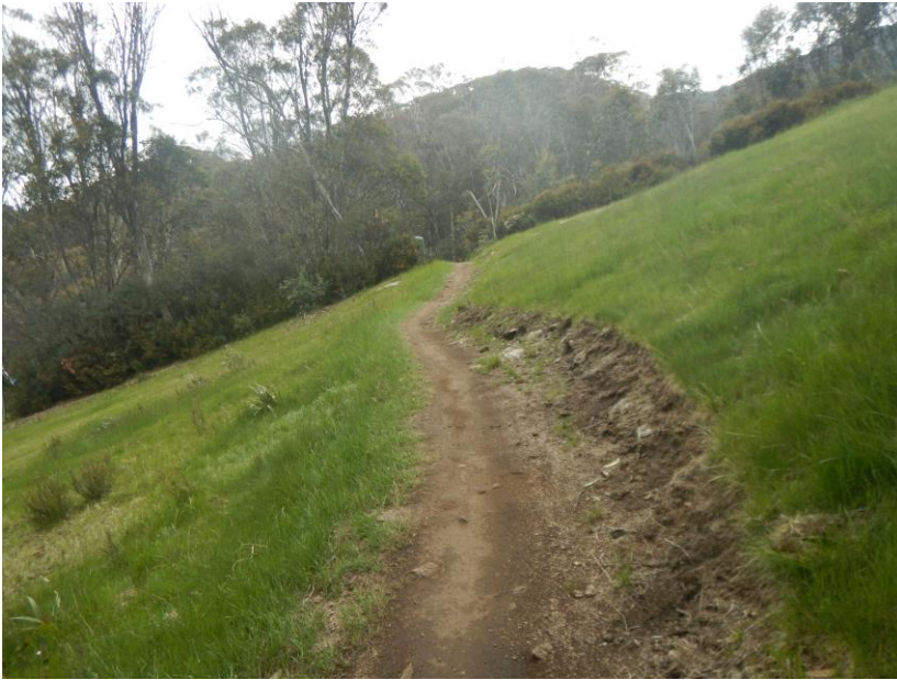
Figure 3 - Existing All Mountain Trail on High Noon - with large cuts impeding summer and winter access
